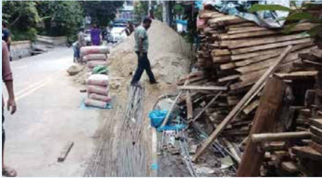
Main road occupied by Construction Material
