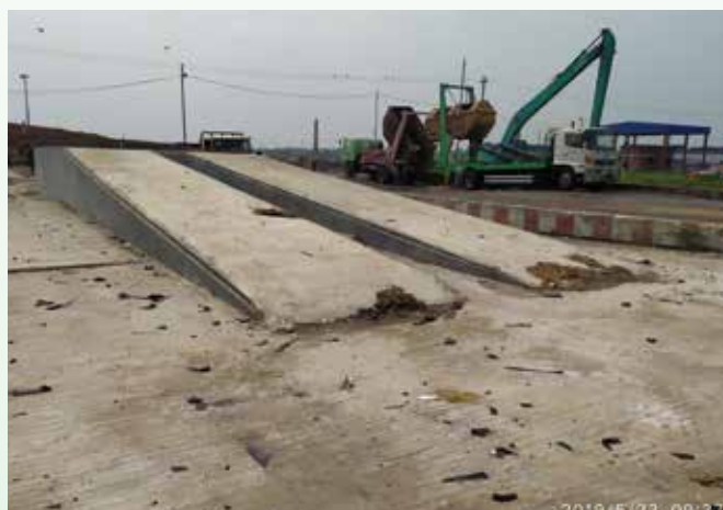
New Car Washing Ramp beside the Car Wash Pool
