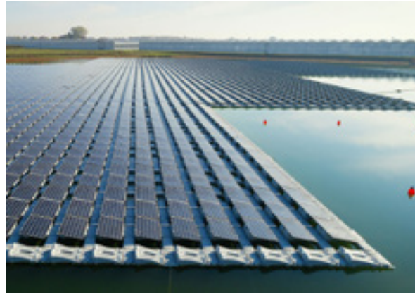
Figure 5.13: Floating PV array based on a modular plastic system which is relatively easy to implement, but possible negative ecological effects
