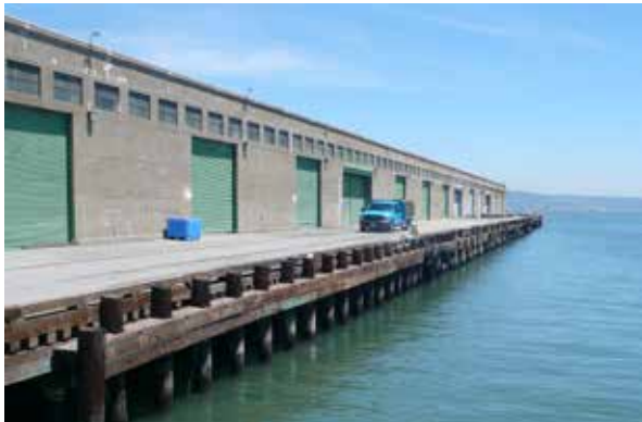
Images of the historic Pier 48 - among three that are threatened by sea level rise in this neighborhood.
