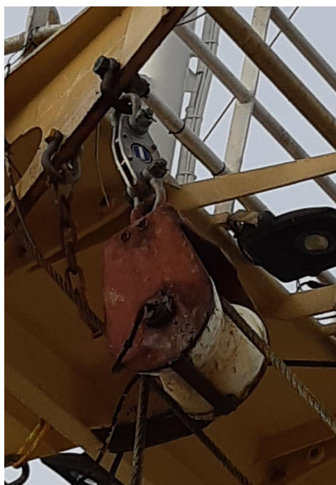
Figure 4: Load cell with safety plates mounted between mast and jumper block. Photo: Tom Bangma
