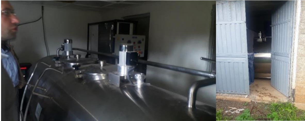
Figure 4 2m 3 cooling tank in a chilling centre near Derba, Ethiopia.
