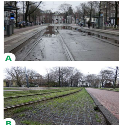
Figure 29 - A - Tram track that has flooding in the Muiderstraat. B - Tram track with permeable soil without flooding near the Hortus Botanicus.
