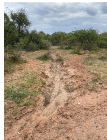
Figure 3: a mitre drain. Photo by courtesy of one of the conservation team’s members.
