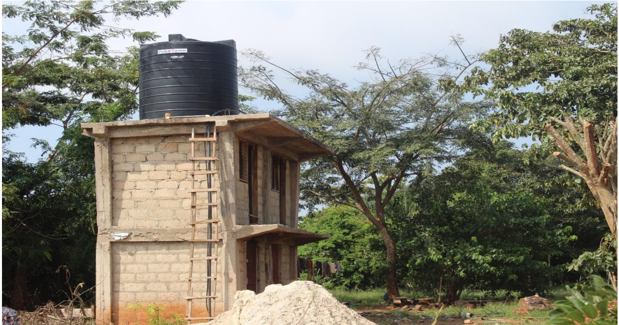
Figure 10: Storage tank for underground water storage for irrigation
