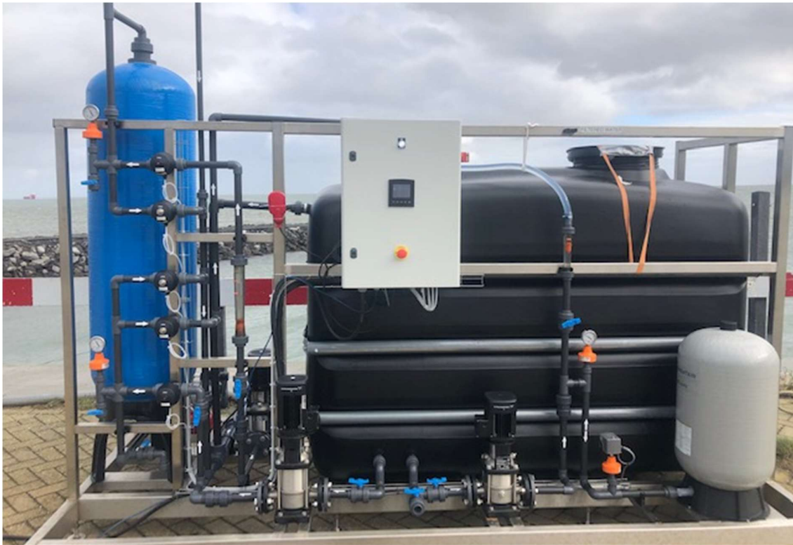
Figure 4: Seawater intake as installed on the dock of Seaport Texel, with the sand filter (blue), 3000 litre buffer tank (black) and automatic valves (orange). Equipped with touch screen for operation
